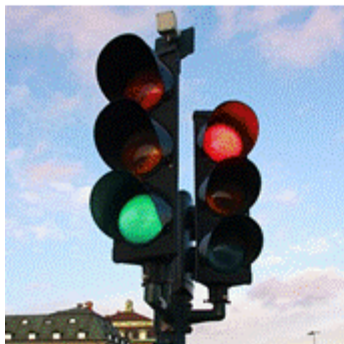
Connected traffic signals
